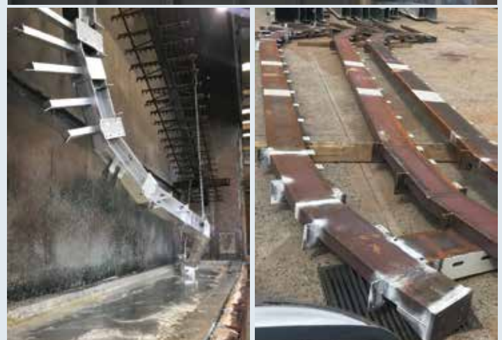
Various members for the main canopies of the five train stations undergo galvanizing.
