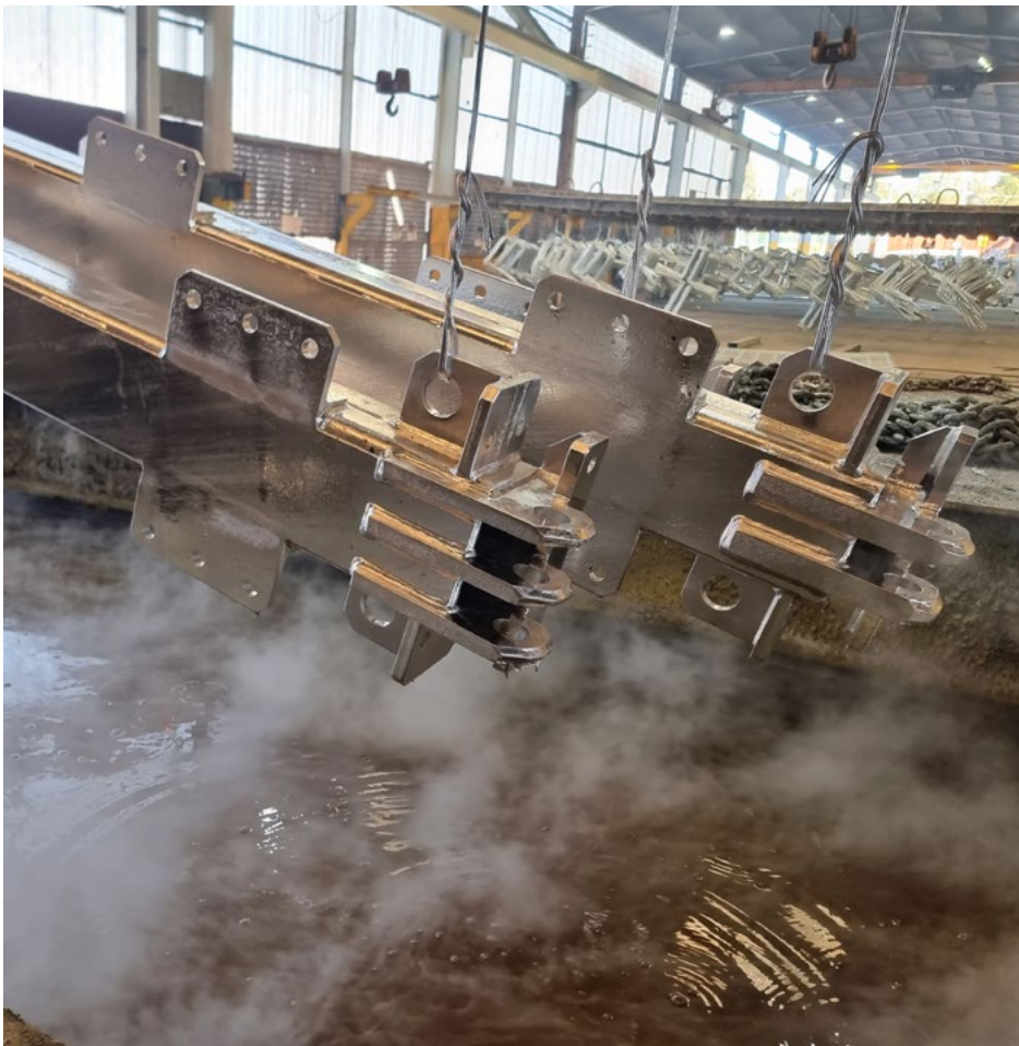
Considering the design and tight tolerance for the pin, meticulous planning, development, and testing of the hot-dip galvanizing process was undertaken.
