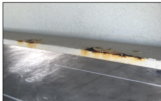
Figure 4: Localised rusting of the structural beam flange under the paint film.
