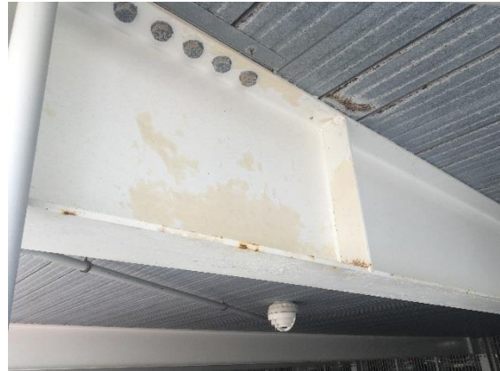
Figure 13: The topcoat of paint seemed to be peeling off the intermediate and the formwork rusting, consistent with water leaking through the concrete.
