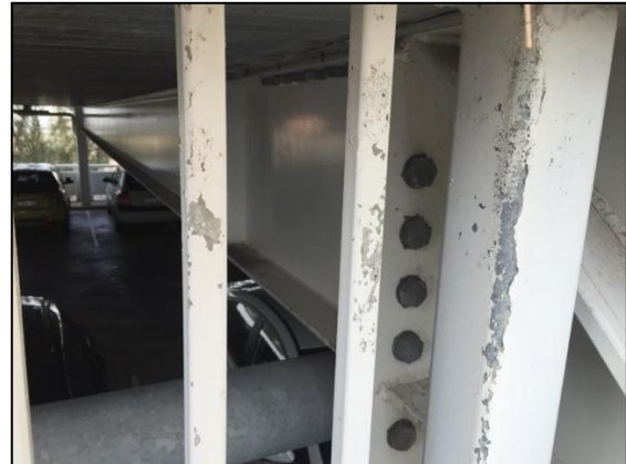
Figure 5: Paint adhesion of the duplex system failing but showing no signs of steel corrosion.
