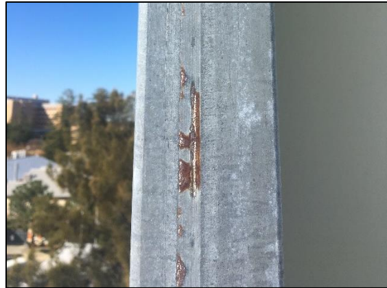
Figure 9: The weld line along the fabricated SHS was corroding earlier than the surrounding galvanizing, indicating an inadequate automatically applied initial repair.
