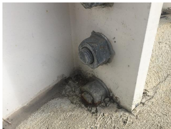
Figure 14: Fasteners have been embedded in concrete on the top floor, leading to ponding of water, crevice corrosion and difficulty when repair is required.
