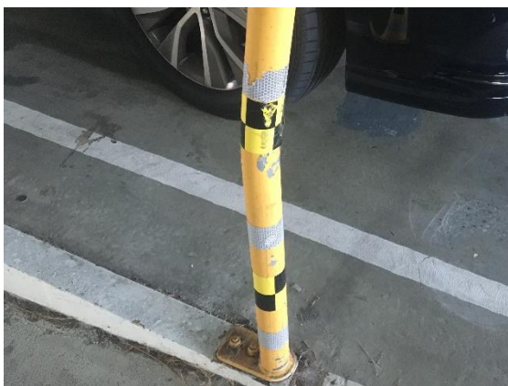
Figure 12: The impact from a vehicle has removed areas of paint, however the galvanizing is still intact and protecting the base steel.
