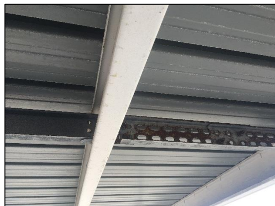
Figure 8: The in-line galvanizing that was sheltered and closest to the coast showed worse signs of corrosion, with an adjacent member slightly further from exposure having no visible red rust.
