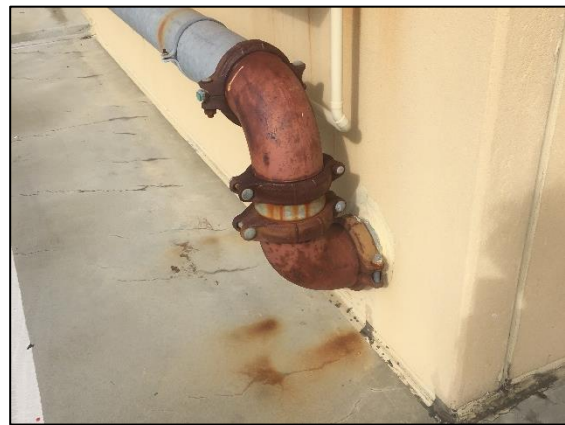
Figure 11: Curved pipe sections to supply water to fire hoses seemed painted only, with rust staining on the ground underneath from corrosion.
