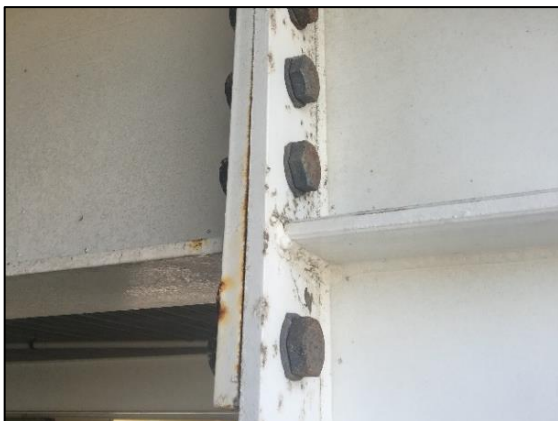
Figure 7: Exposed joints gave a direct comparison between using paint only, duplex systems and HDG to protect the steel when exposed to the same environment. The duplex system protected the base steel although the paint had lost adhesion in some areas. The HDG fasteners had white rust in places, formed by the natural corrosion of the zinc coating but no signs of corrosion of the base steel. The paint only sections showed areas of heavy corrosion of the base steel in some areas, with red rust clearly visible and filiform corrosion likely.
