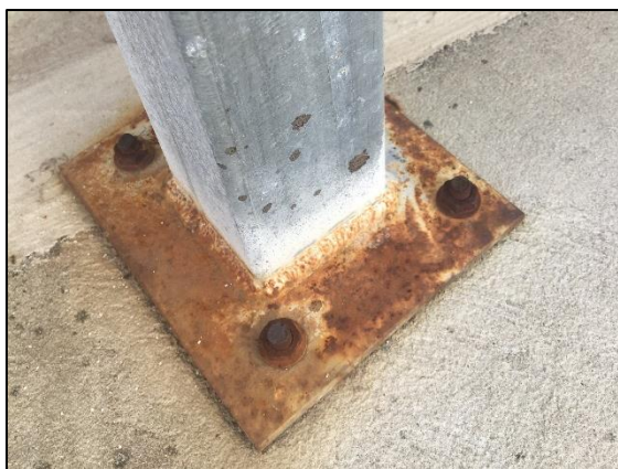
Figure 10: A painted base plate welded to galvanized SHS has corroded, with ponding of water potentially increasing the corrosion rate.
